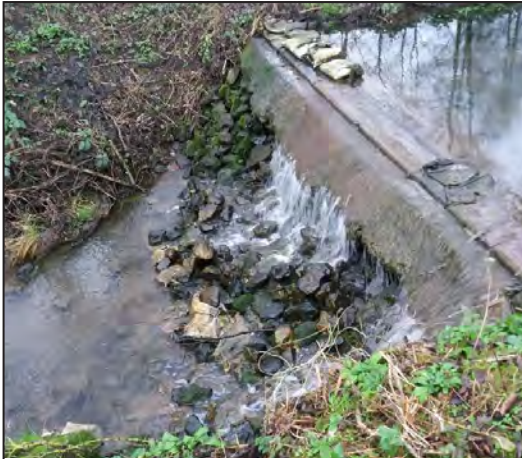
The current weir at Pinxton showing concrete top with loose stones below.
