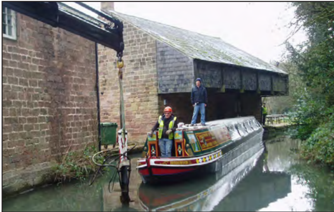
Removing the rudder (which houses the propeller and failing motor) from Birdswood. Photo: John Baylis
