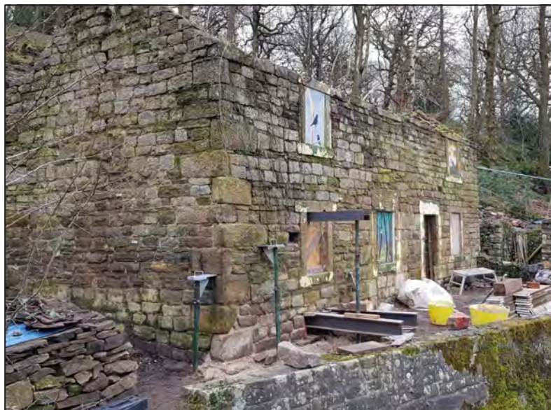
Work is progressing rapidly on stabilising Aqueduct Cottage at Leawood, helped on by a £6,000 grant from FCC. Photo: Ron Common
