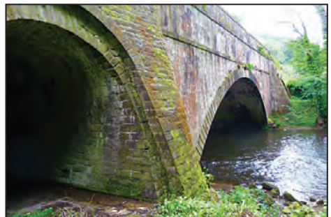
The view of the north-eastern face from below Aqueduct Cottage clearly shows the difference in construction of the three arches.
