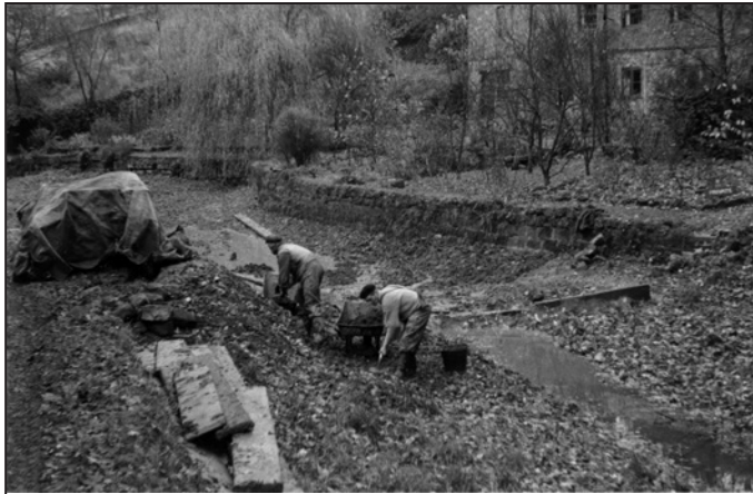
During 1945–47 extensive work was needed to repair the culvert carrying the water of the Leashaw Brook under the canal.
