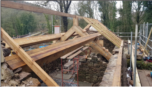
The massive purlins can be seen along with details of other timber work.
