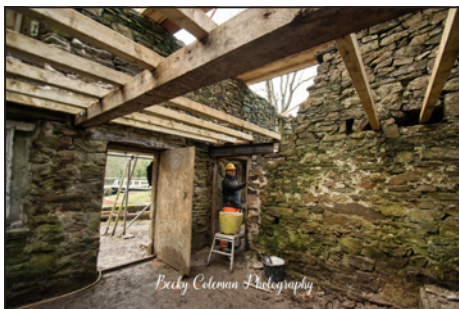
The beginnings of the floor transforms the interior. The steel beam connects the central internal wall to the front wall.
