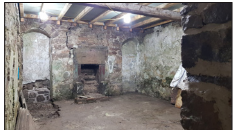
With the floor above in place, the interior is looking homely with its original fireplace.
