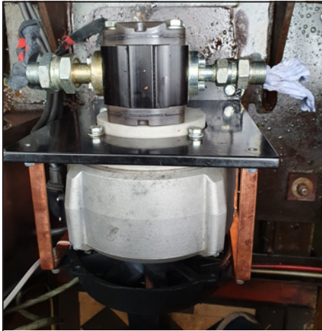
The reinstalled motor/pump unit with fan attached, awaiting recoupling of the hydraulic hoses.
