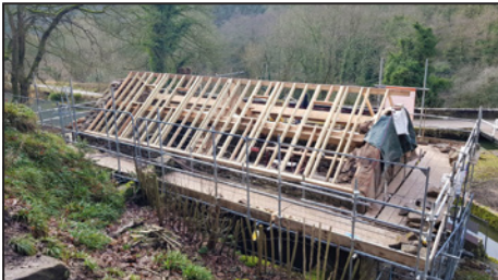
The roof takes shape with the spaces for the Velux windows visible.
