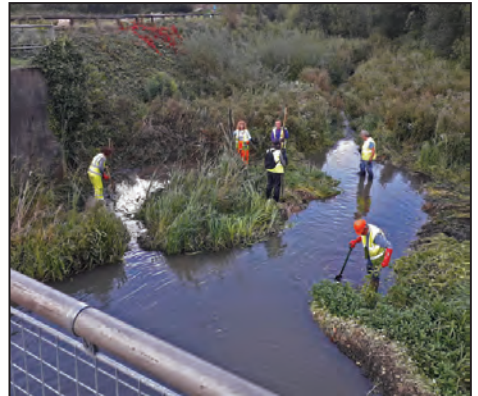
Clearing the remarkably wide channel of the Codnor Park Reservoir overflow at the request of CRT.
