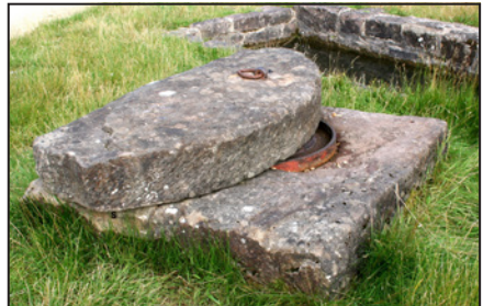
The pad-stone in position. (The lump on top has nothing to do with the bridge!)
