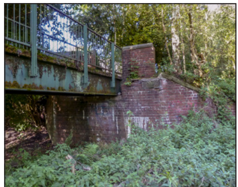
Study of the abutments shows that they were built for a much wider deck than is currently in place. Does anyone recall when this work was done
