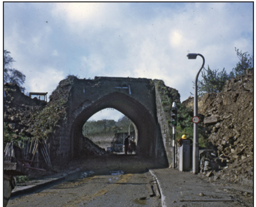
A pause in the demolition allows a family with small children to pass under the half-destroyed arch.
