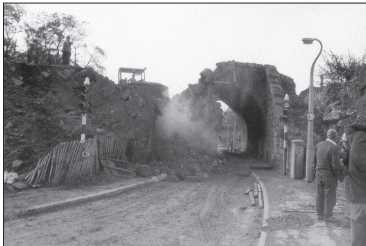
Demolition of the aqueduct underway, without the aid of barriers to keep the public out.
