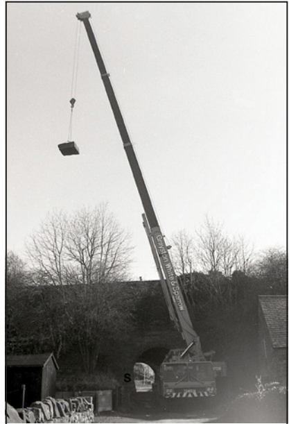
The crane's 90ft jib lifts the pad-stone away and down to the lorry.
