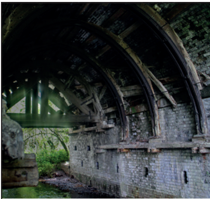
The rather decayed second bridge/culvert under the derelict Mansfield & Pinxton railway line, built around 1819.
