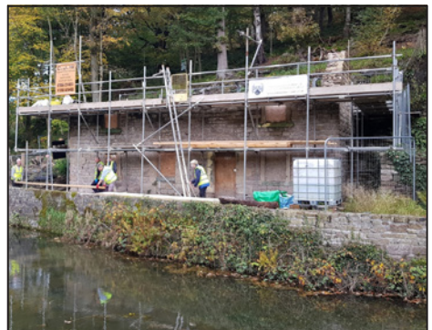
The timber finally arrives at Aqueduct Cottage ready to be used to build the roof structure.
