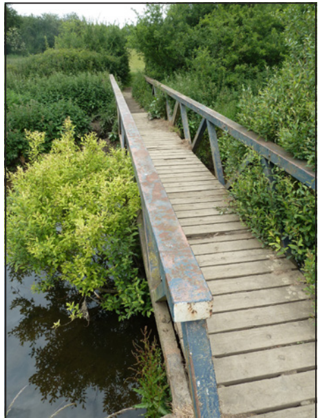
The overgrown footbridge on the site of the aqueduct across the Erewash below Stoneyford.
