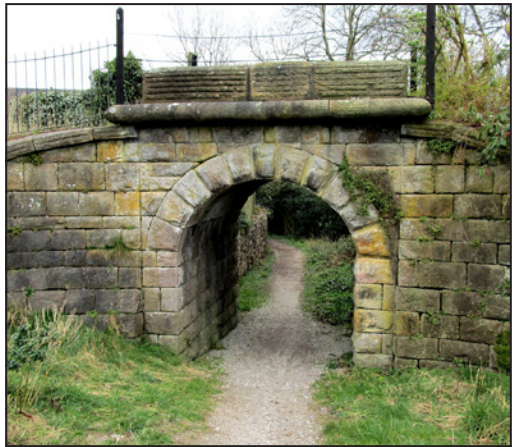
Bridge at Coasthill for the Crich Railway built by George Stephenson in 1841 to carry limestone from the quarry to his kilns at Bullbridge.
