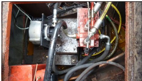
The complex system of hydraulic pipes that operates the boat's electro-hydraulic system. The defective motor is on the left.
