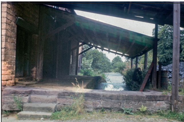
Not only was the canopy still present on the Gothic Warehouse but there was a second canopy at a different angle over the entry door. Note the coal in the yard to the right.
