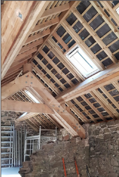
The exposed roof structure provides great character to the first floor activity room.
