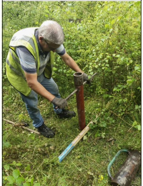
Taking core samples in preparation for the Beggarlee Extension. The bridge is the former Barber Walker Colliery Railway bridge that the new line of the canal will pass through.
