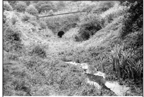
The western portal of Butterley Tunnel as it appeared before the A38 was built across it.
