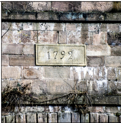
On the downstream side of Derwent Aqueduct is the optimistic date of 1792. In fact there are two such dates: the more prominent one appears to be a later addition to the earlier one carved into the stone below it. This date presumably reflected the initial completion of the structure.
