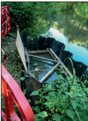
Shallow piling sealed off the recent leak at Robin Hood whilst awaiting repair.
