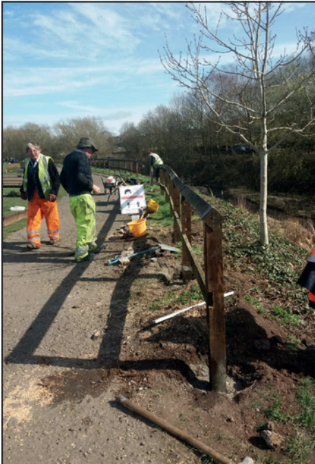
The repaired fence at the site of Lock 1 which had been destroyed by CRT contractors.
