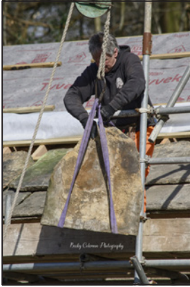
Lifting the stone tiles weighing up to 60kg was assisted by a pulley. Photo: Becky Coleman
