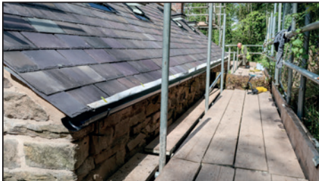
Replacing the guttering at the rear. Photos by Ron Common unless credited
