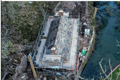
A drone's eye view of progress showing the completed roof. Photo: Andrew Woodward
