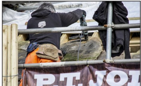
Modern tools help to fix the stone tiles in place. Photo: Becky Coleman
