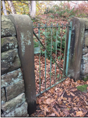
One of the many gates that once gave access to the pipeline, apparently never now used.
