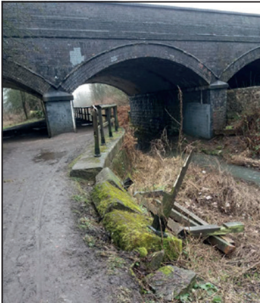
The displaced coping stones above the railway bridge.
