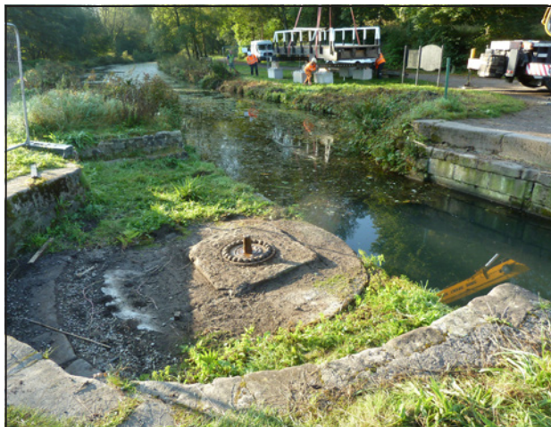
The old bearing and pintle showing the swinging area for the bridge, which is being positioned on its 'Lego' blocks in the background.
