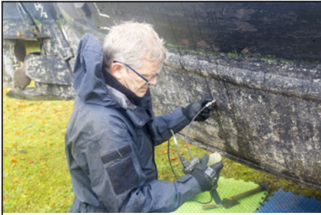
Our surveyor, Adrian White, taking thickness measurements near the stern. Photo: Keith Bailey
