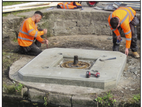
Reuben and Josh finishing the concrete base for the new slewing ring.
