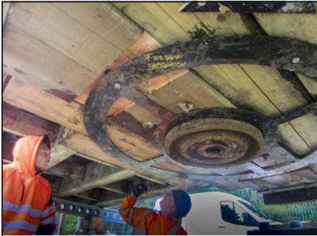
Foreman Steve using the upper template to accurately position the required drill holes. The top half of the original bearing ring is in the centre.
