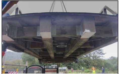
The underside of the bridge deck being swung across the canal showing the new bracing bars and other stiffening works added.
