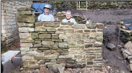
In the wash house! Rebuilding the small outbuilding next to the cottage.
