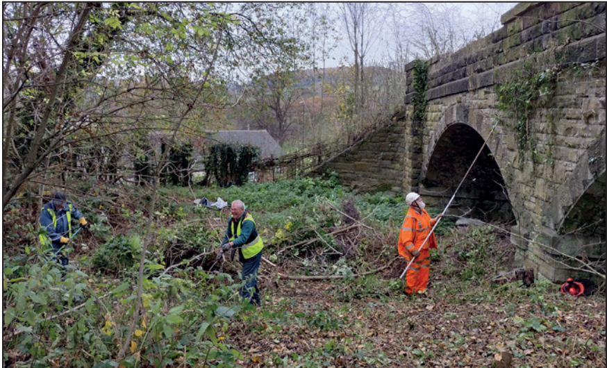
Attacking the rampant vegetation at Brickyard (aka Lockwood's) Bridge, Sawmills. Note the missing parapet stones, which are still to be found..
