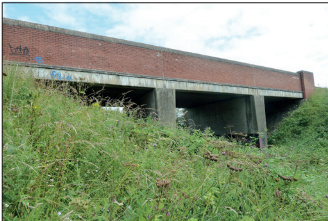
The former Barber Walker colliery railway bridge through which the new canal will pass under the A610.
