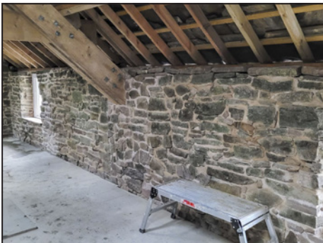
After lime mortaring. One of the interior walls will be left unplastered to show the original stonework.
