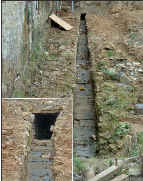
The newly exposed culvert looking up to the canal bank. Inset: A glimpse into the section of culvert still beneath the canal.
