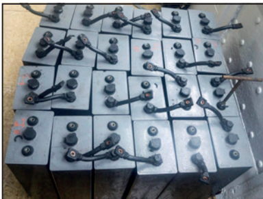
Birdwood's 24 805AH cells disconnected awaiting loading for reconditioning.
