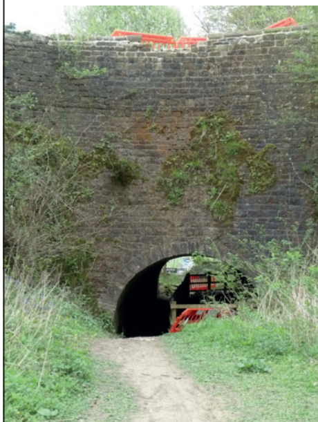
The parapet above Buckland Hollow Tunnel was once again damaged by traffic, causing the temporary closure of the towpath beneath, happily now reopened.
