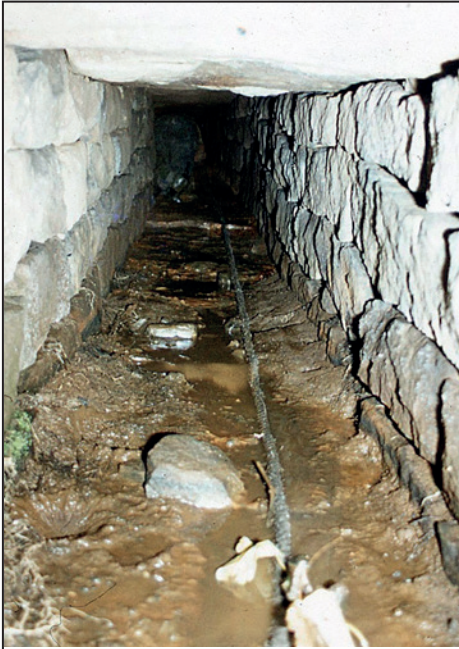
When Simon Stoker's team investigated the culvert at Gregory Wide, they took this remarkable photograph showing its confined size but perfect stone construction. The rope was a safety rope.
