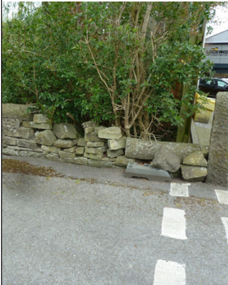
The parapet of the original Brickyard Bridge at Sawmills (adjacent to the 4-arch bridge by Lockwood's entrance) is in dire need of TLC which it is hoped the lime-mortar-trained work party will be able to gain permission to do.
