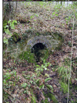
. . . and the outlet from the culvert which led to a second culvert taking the water under the adjacent railway.
