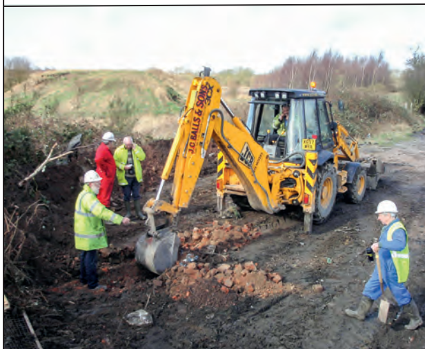
John Baylis directs operations at the first work on the Smotherfly site, work that was subsequently made impossible through the demise of UK Coal and its promised finance.
