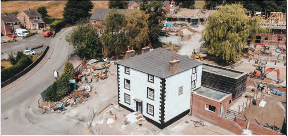
A drone's eye view of the Canal Inn under restoration and the new houses being built behind it.
