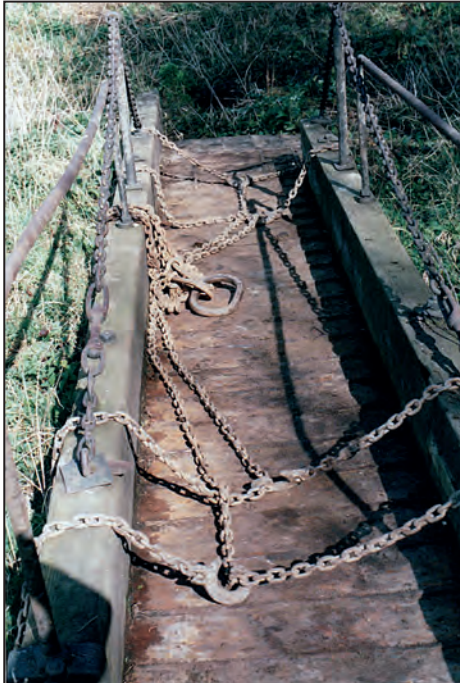
The bridge awaiting lifting, with the ridges in the cast iron decking visible.
