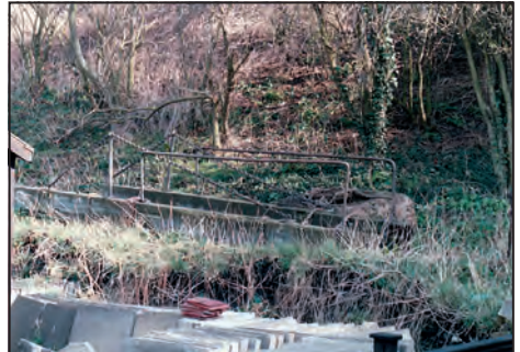
Having been craned from their original location on top of the aqueduct, the bridge and pivot stone were placed alongside Drovers Way to be craned onto the low loader.
