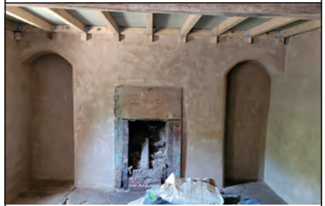
Elegant arches on either side of the parlour fireplace after their second coat of plaster.
