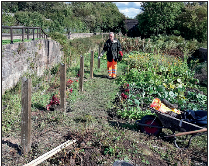
FCC volunteers erected safety fencing between the garden and the lock chamber in 2017.
