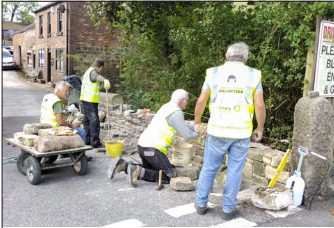
Progress as the bulk of the wall is rebuilt. Waterloo Farm is the brick-built building in the background.
