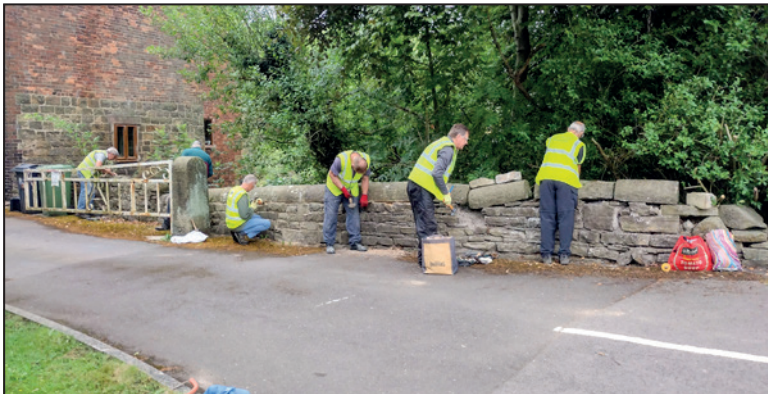
Work begins on the rapidly collapsing wall.
