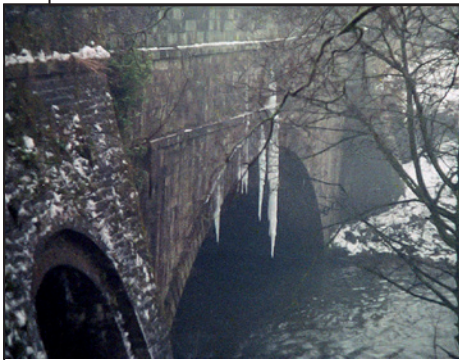
Before the aqueduct was lined with rubber sheeting, it regularly leaked, which showed up particularly well in winter!
