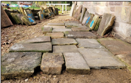
A rather heavy jig-saw to test the layout of the reclaimed stone flags.
