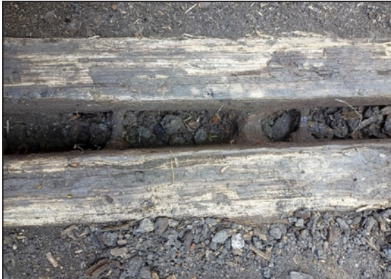
A close-up of the two base planks with metal fastenings between. It is thought that a third, raised, stop plank was positioned here to give a base that would be free of debris to take the other planks.
