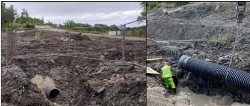
The pipes that FCC volunteers have fitted and the position at the end of August, with 45m of pipework laid.
