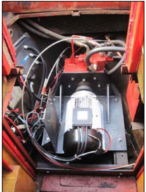
Our original electric motor installation (now replaced).
