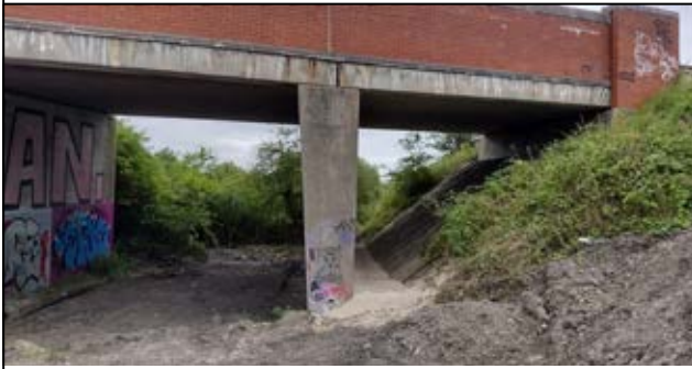
The footpath has been laid through the bridge to the right of the right-hand pillar.
