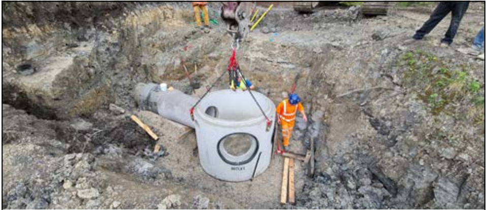
Large scale work has now begun at Beggarlee placing a large concrete manhole.
