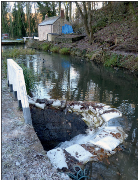
A temporary dam surrounded the sluice at Leawood whilst the paddle was replaced.
