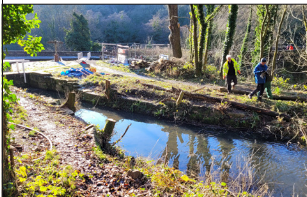
The exposed stop lock chamber and the badly damaged and displaced coping stones.
