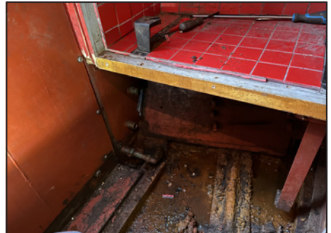
Hull brace under the stove shortly after exposure. Note the corrosion and slime.
