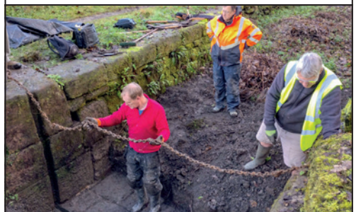
The chain discovered in the infill could well have been used to prevent boats passing without paying tolls.
