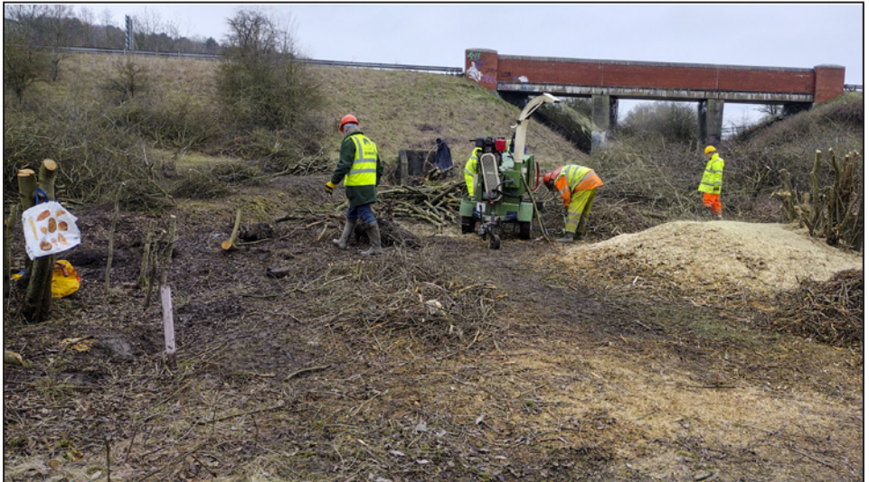
Plenty of brush to chip, with the A610 bridge in the background. It is through this former railway bridge that the canal will pass.
