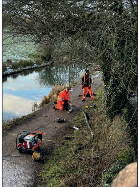
Geopolymer being pumped into holes drilled into the towpath where voids had been detected just north of Lawn Bridge.
