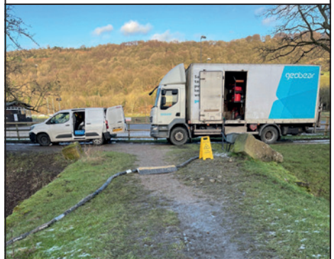
The only access to the site was from the rugby club road. A long pipe was then run to the work site.
