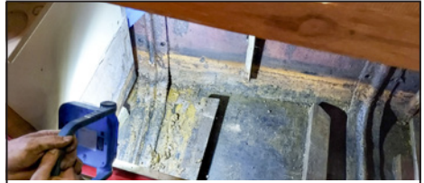
The area below the bed in the boatman's cabin before cleaning.
