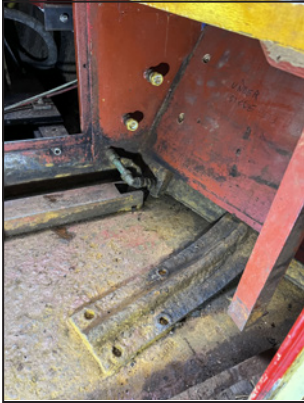
The area under the stove after extensive cleaning.
