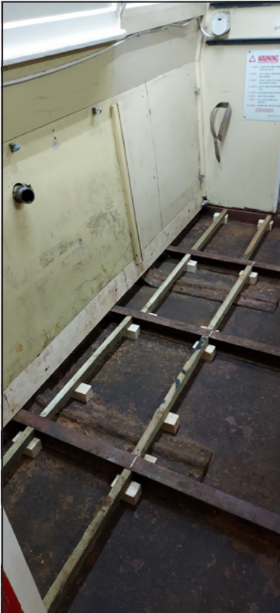
New support battens and now-replaced rotten plywood on the vertical section in the galley
