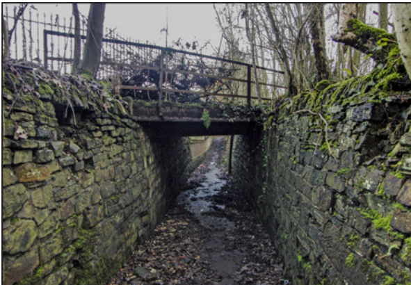
A former rail bridge over the footpath at the bottom of Spring Lane.
