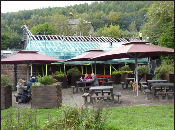
Work on the roof of the High Peak Junction workshops began in October and should be finished before Christmas. During this time the shop/café and toilets remained open.
