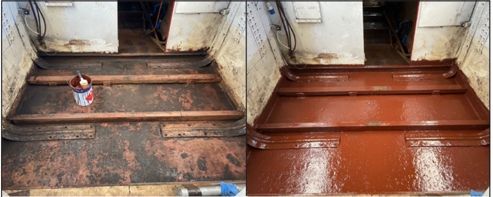
Once the floor plates were lifted and the battery boxes moved, the bottom plates were cleaned and repainted.
