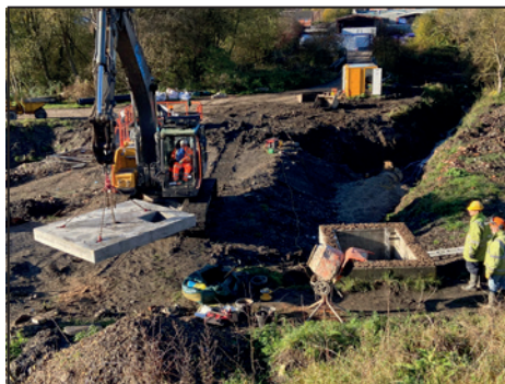
WRG helping to fit the top slab on the headwall of the 900mm pipe at Beggarlee on Remembrance Day.
