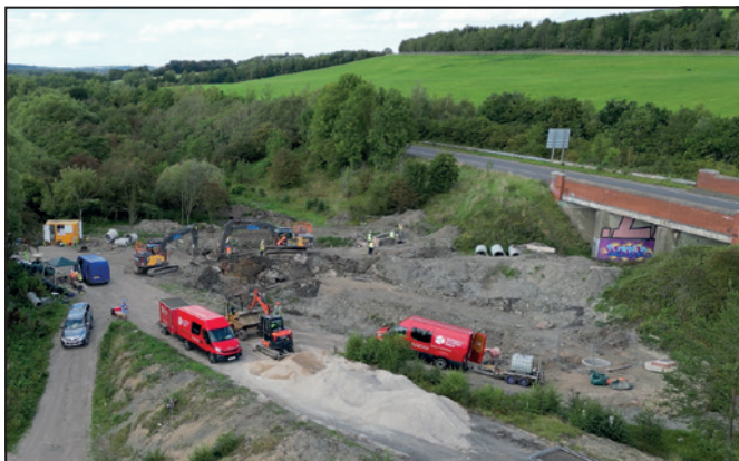
A screenshot from drone footage made during a WRG visit to the Beggarlee site. The former railway bridge under the A610 on the right is where the canal will pass after being raised by a staircase pair of locks at the bottom right of the image.
