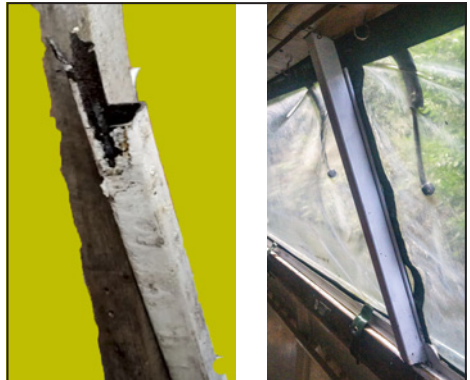
The rotten gutter and the new fabrication made by Malc Chisnell.
