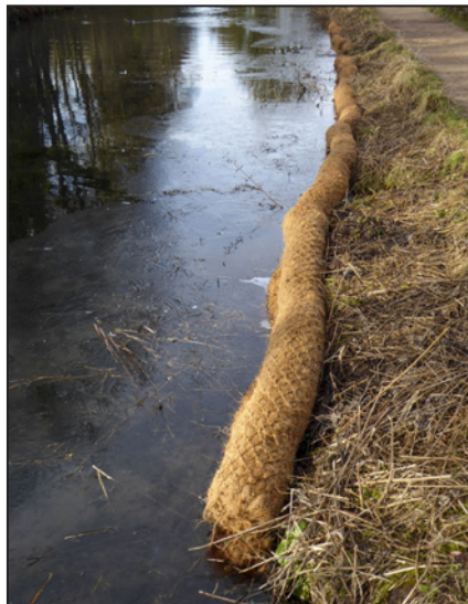
Coir rolls newly inserted for bank protection by Brown's Swing Bridge at High Peak Junction.
