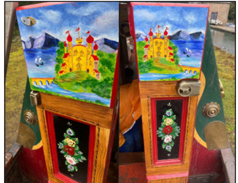
The original decorative wooden inserts in the steel rear doors at the rear entrance to the boat were extensively rotted and needed complete replacement. Ian Hutchinson made and fitted exact replacements together with the new mortice lock.
