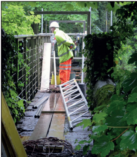
Repairs to the footbridge across the River Derwent on the route to HPJ.
