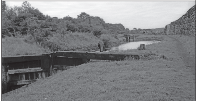
Probably taken a few years after Mr King's visit, the top gates of Lock 2 are still, just, holding water, but the balance beam has broken. The bottom gates of Lock 1 are bare framework. The high wall Mr King referred to is on the right and was made of slag from the Butterley Co furnaces.
