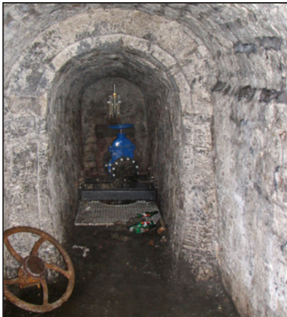
The valve set into the dam wall of Butterley Reservoir that releases water into the tunnel beneath.
