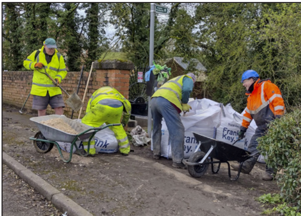
Transferring the granite chippings from the road bridge to the work site.
