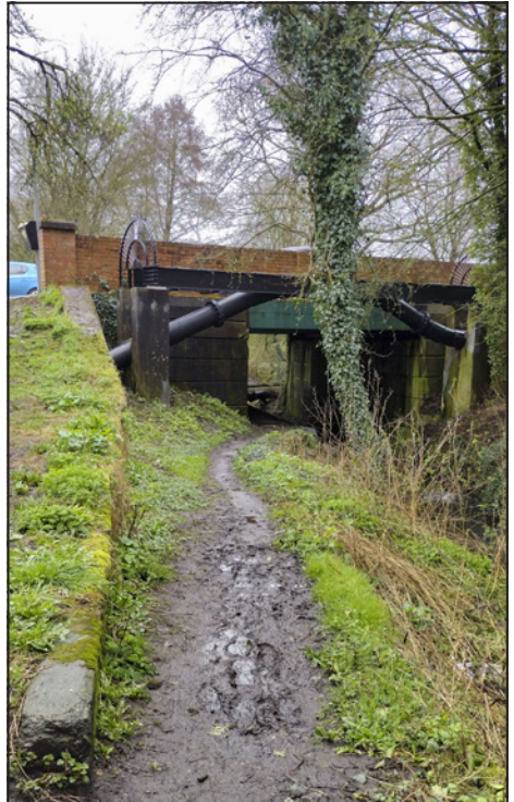
The poor state of the towpath before work began.
